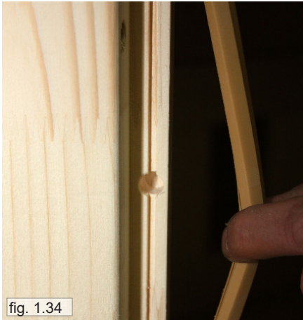
Door seal from the glass door
